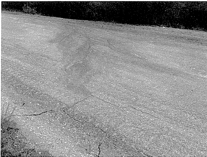
Light erosion and sediment deposition on a roadway.
