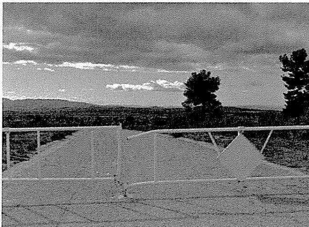
Vehicular gate in need of repair.
