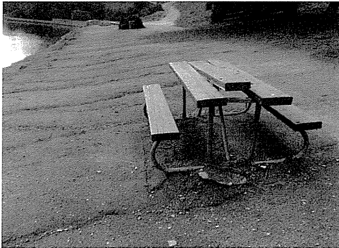
A picnic table in need of repair.
