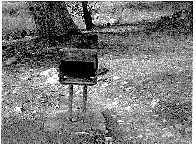
Erosion around the base of a barbecue pit.
