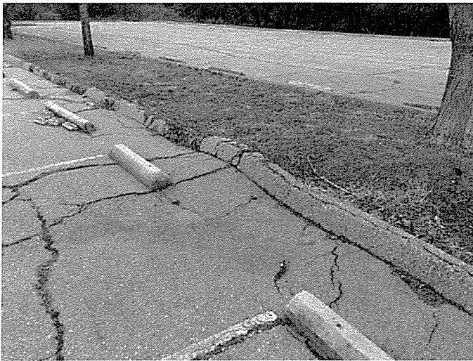
Example of the damage done to asphalt parking lot/curbs from adjacent trees, this will need to be rebuilt.
