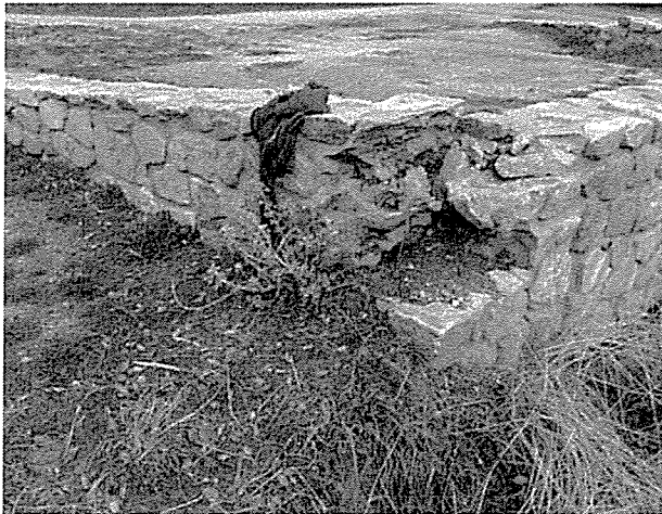
Stone on wall in need of repair/ replacement.
