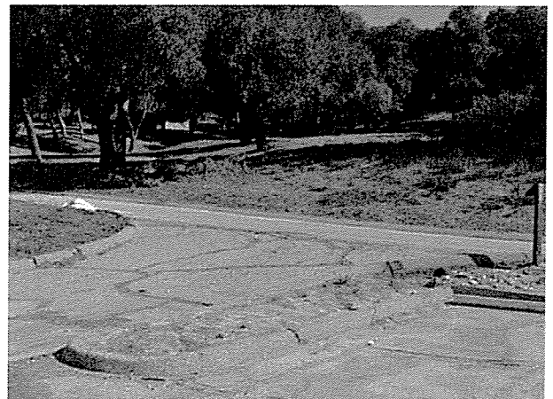
Example of the pavement and curb with erosion control repairs that are required.
