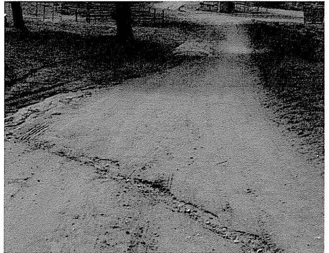
Erosion/drainage issues along the dirt roads.
