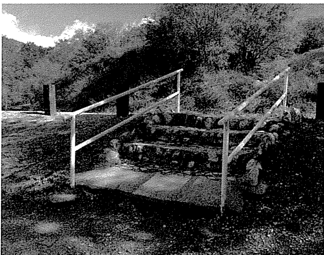
The base of the landing requires fill soil.
