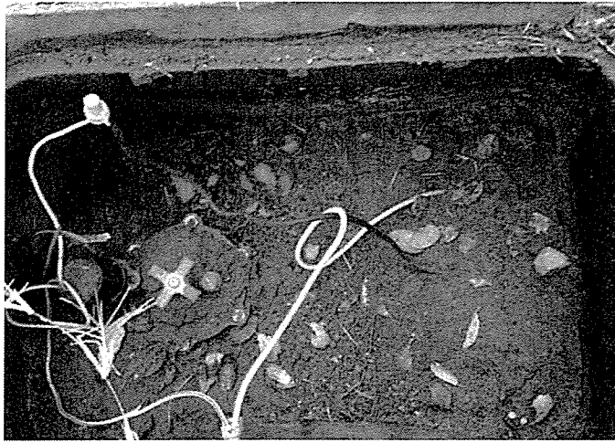
Sediment filled irrigation control box.
